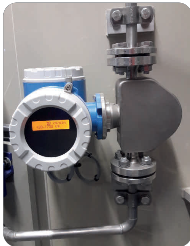
Detail of the polymer solution station AWV Grazerfeld
