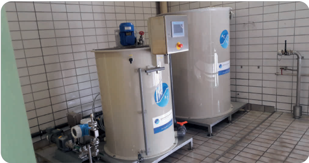
AWV Hall Tyrol – Fritzens Polymer dissolving unit FPU for sludge dewatering with belt decanter
