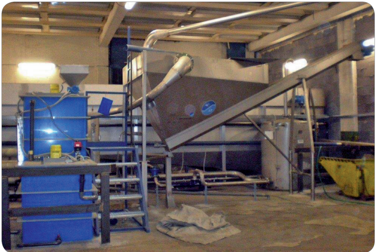
The caustic solution is neutralized with AluStar® products to clean the waste water.
