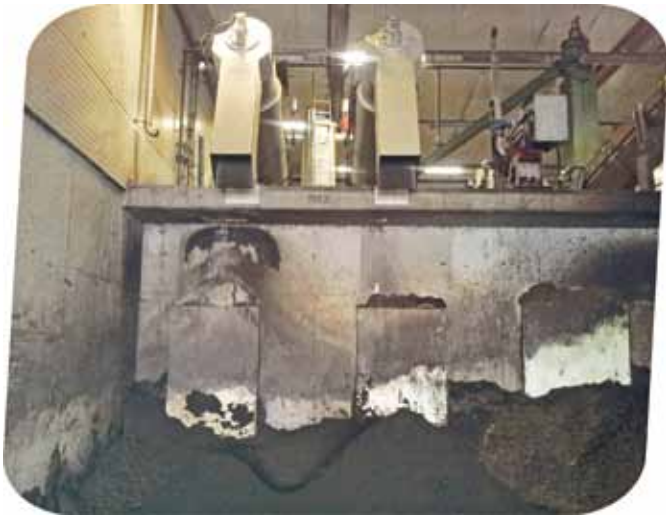
Dewatering of fermentation residues with flocculants from ACAT with two screw presses (please also have a look at the picture on the left-hand page)
