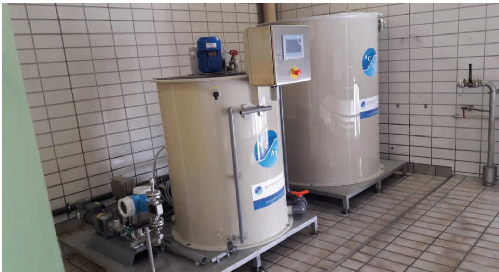
AWV Hall Tyrol – Fritzens Polymer dissolving unit FPU for sludge dewatering with belt decanter
