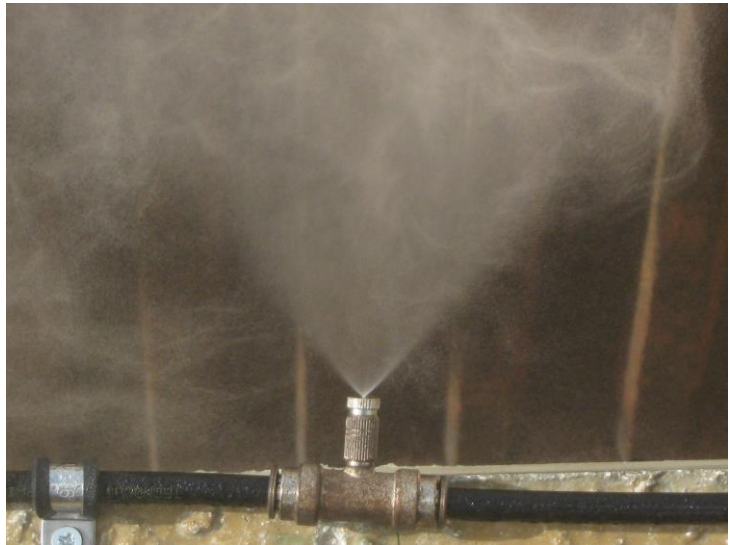
A spraysystem was installed; the picture shows a nozzle detail
