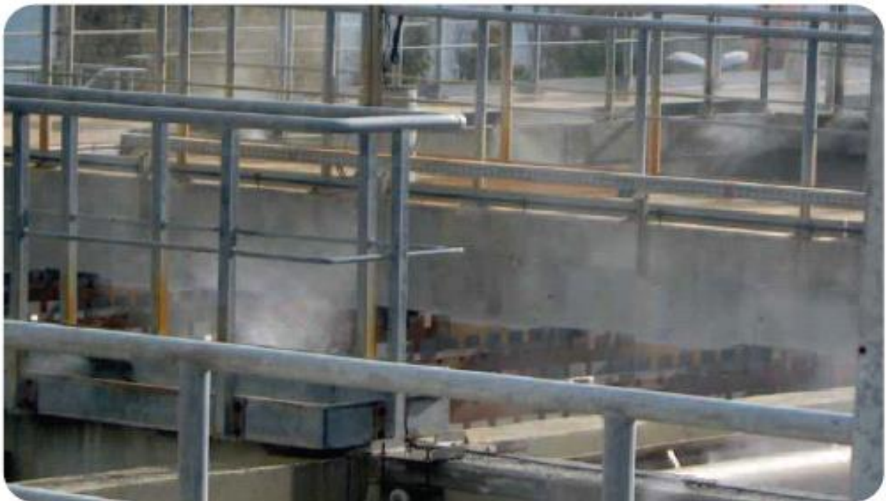
In Malta Waste Water Plant we installed a High Pressure System to dose ECOSORB® 606
