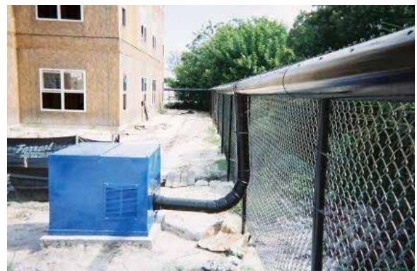
Ecosorb® Vapour Phase Equipment used at a site perimeter.
