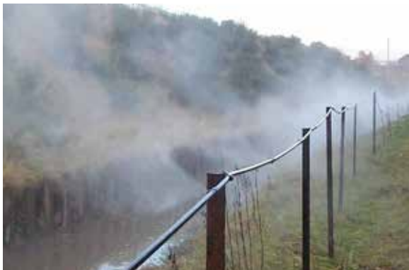
High-pressure nozzle line used to atomise Ecosorb® during diffuse odour situations.
