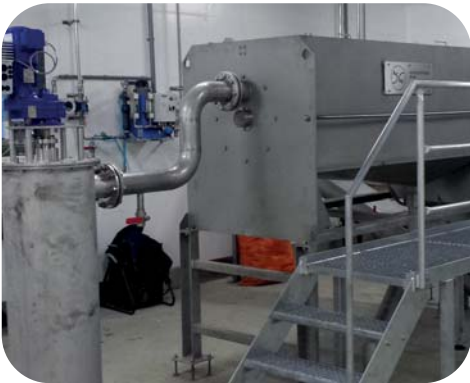
Top upgrade of the wastewater treatment plant Ariolo in Ticino with ACAT-screw press type AS 450
